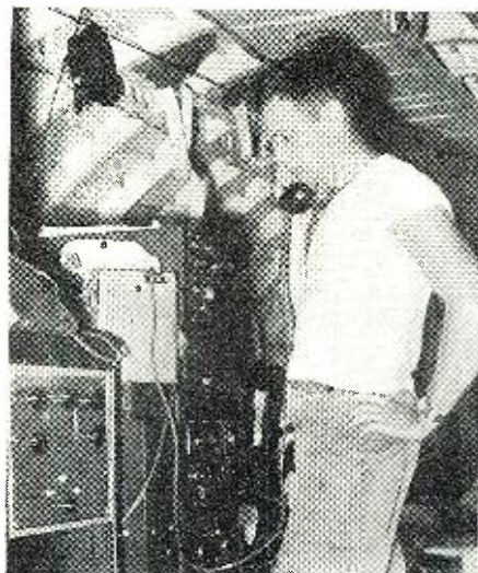
Interior of transmitter plane, showing 3 kw. radioteletype transmitter, frequency shifter FS 112A, and transmitter BC 610 (Hallicrafters HT4).
